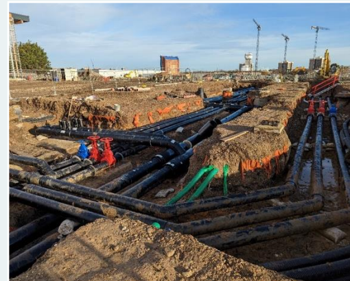
Underground connections for a commercial plot
