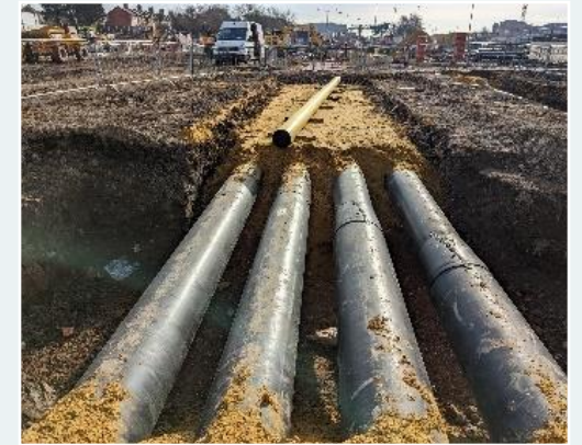
Heating and cooling pipework
